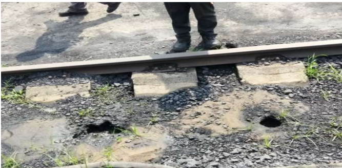
Fig. 8: Formation of holes near rail track due to water percolation of Fire hydrant
