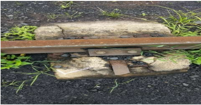
Fig. 7: Disintegration of rail track concrete
