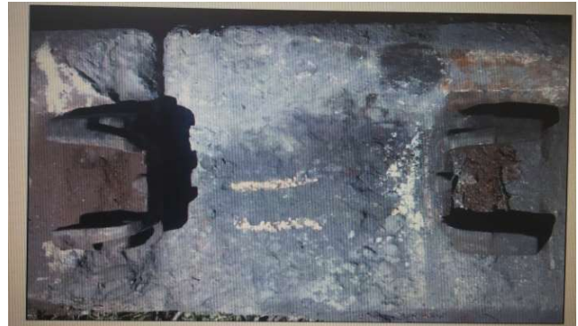
Figure 2.7 Example of concrete-tie rail seat deterioration (RSD)
