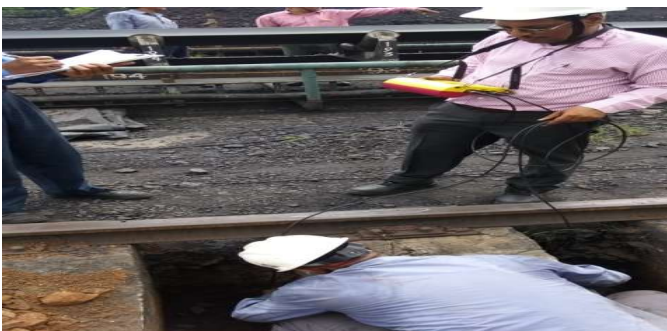
Fig.10 Ultrasonic test of rail track RCC foundation of stacker reclaimer in CHP
