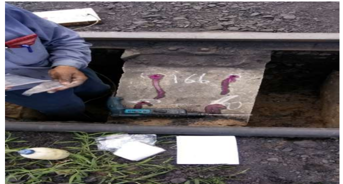
Fig.11 Carbonation test on RCC Rail track foundation of stacker reclaimer
