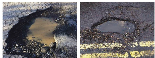
Fig. 1 Images of Potholes on Road
