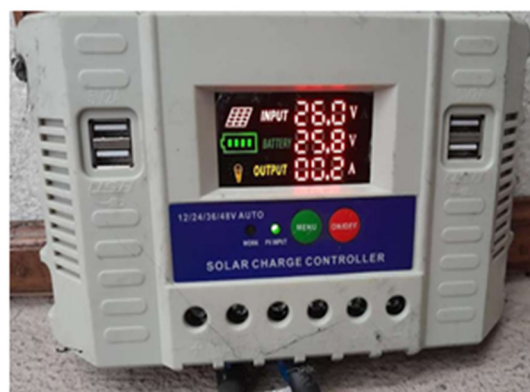
Fig.1. MPPT and solar charge controller for measuring the short circuit current, open circuit current, maximum current, maximum voltage and maximum power.
