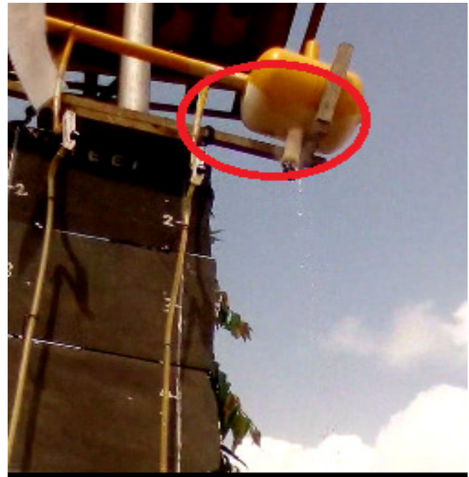
Figure 9: Condensed multiphase fluid from the vent section exit.
