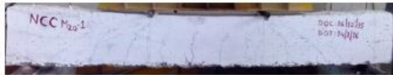
Fig. 5 CRACK PATTERN -II
