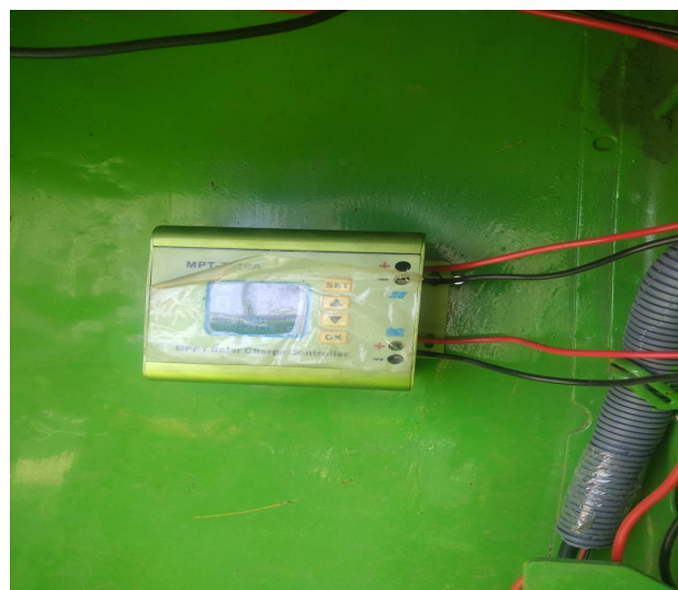
Fig:13 MPPT Installed in SPEV
