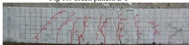
Fig 11. Crack pattern B-4
