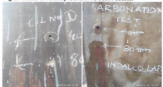
Fig. 6: RCC Columns Carbonation 40mm & 80mm Depth
