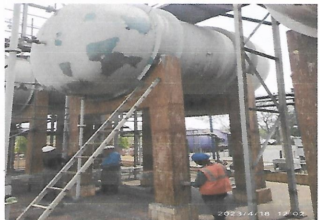
Fig. 5: Cracks & Porosity found in TG deck Pedestal
