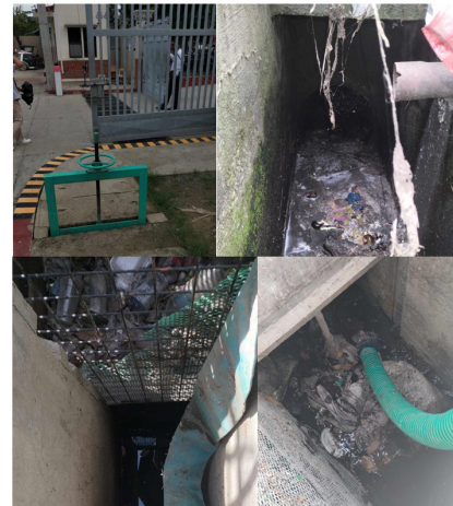
Fig. 12 DHVSU Drainage Outfalls
