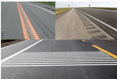
Fig. 1 Types of Rumble Strip – (Up Left) Centerline, (Up Right) Shoulder, and (Bottom) Transverse
