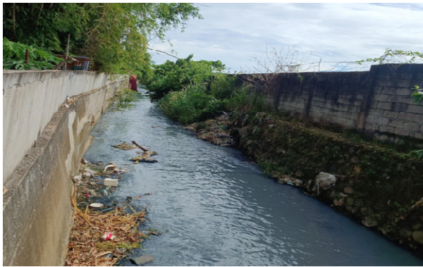
Fig. 3 Slope Rehabilitation Project in Selected Areas of the San Agustin Creek, City of San Fernando, Pampanga
