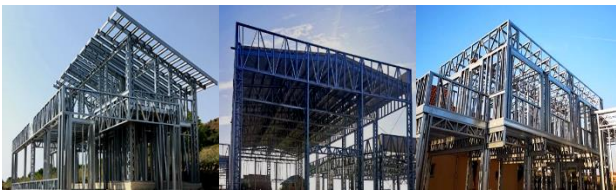
Fig 10. Cold formed steel structures by Mexi Steel using EN 1993
