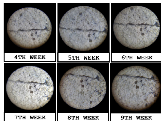
Fig. 1c. Visual observations of closure of crack, Traditional concrete
