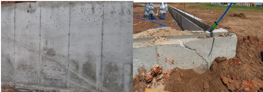
Figure 1. Cold Joint on Reinforced Concrete Structure
