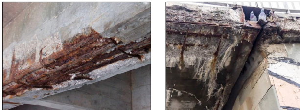
Fig. 1.1.a (left) shows exposed corroded internal steel reinforcing bars in a beam and Fig. 1.1.b (right) shows a totally exposed steel bars in the slab of the structure. (Source: left – Ju-Seong et. al., 2022; right – Corrosionpedia, 2019)
