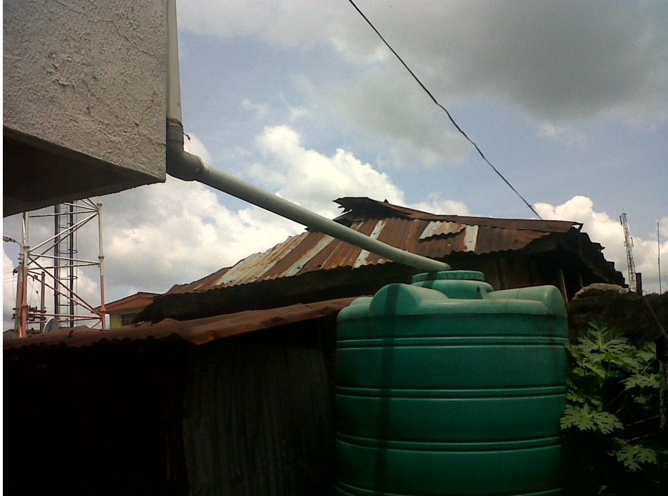
Plate 1: Rainwater harvesting channelled to ground level storage tank.
