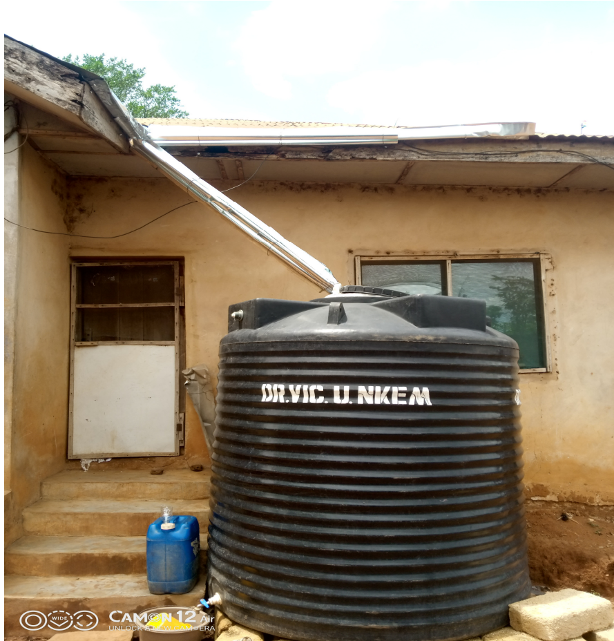
Plate 2: The edges of the corrugated iron roofs are eaved round and channelled to the storage tank.
