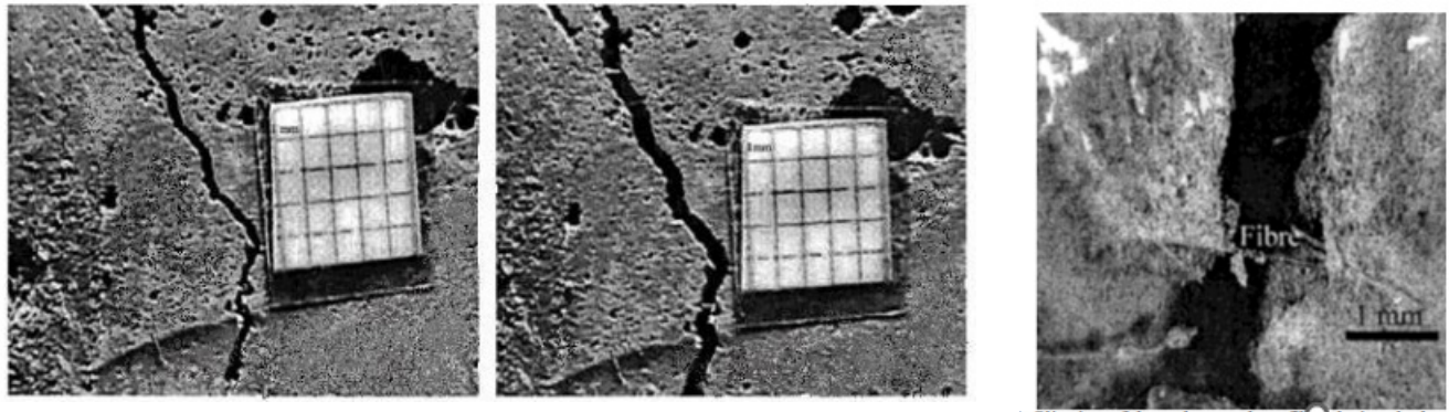
Fig. Crack With width in FRC with 0.1% and 0.3% Polypropylene Fiber.
