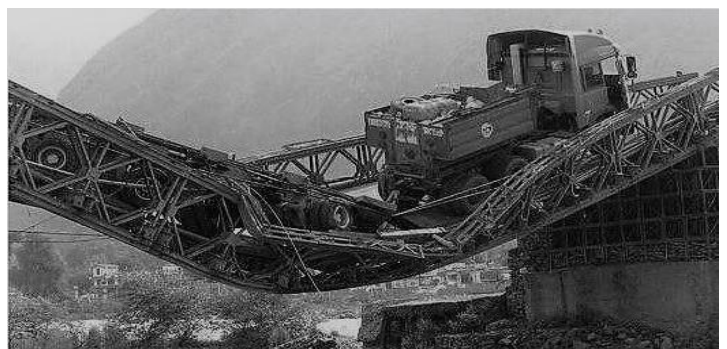
Fig.1 Collapsed Flyover due to overloaded truck.
