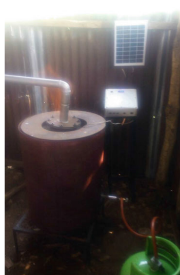
Figure 2: Gas-fired furnace with attached solar-powered temperature sensor
