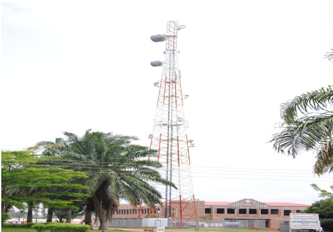
Figure 2 Base Transceiver Station (BTS)
